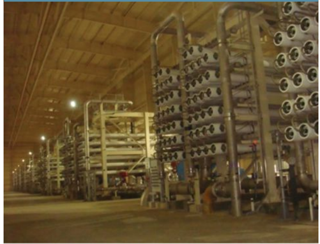
Figure 5. Second RO membrane bank
