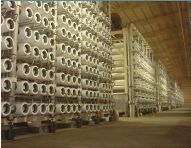
Figure 4. First RO membrane bank
